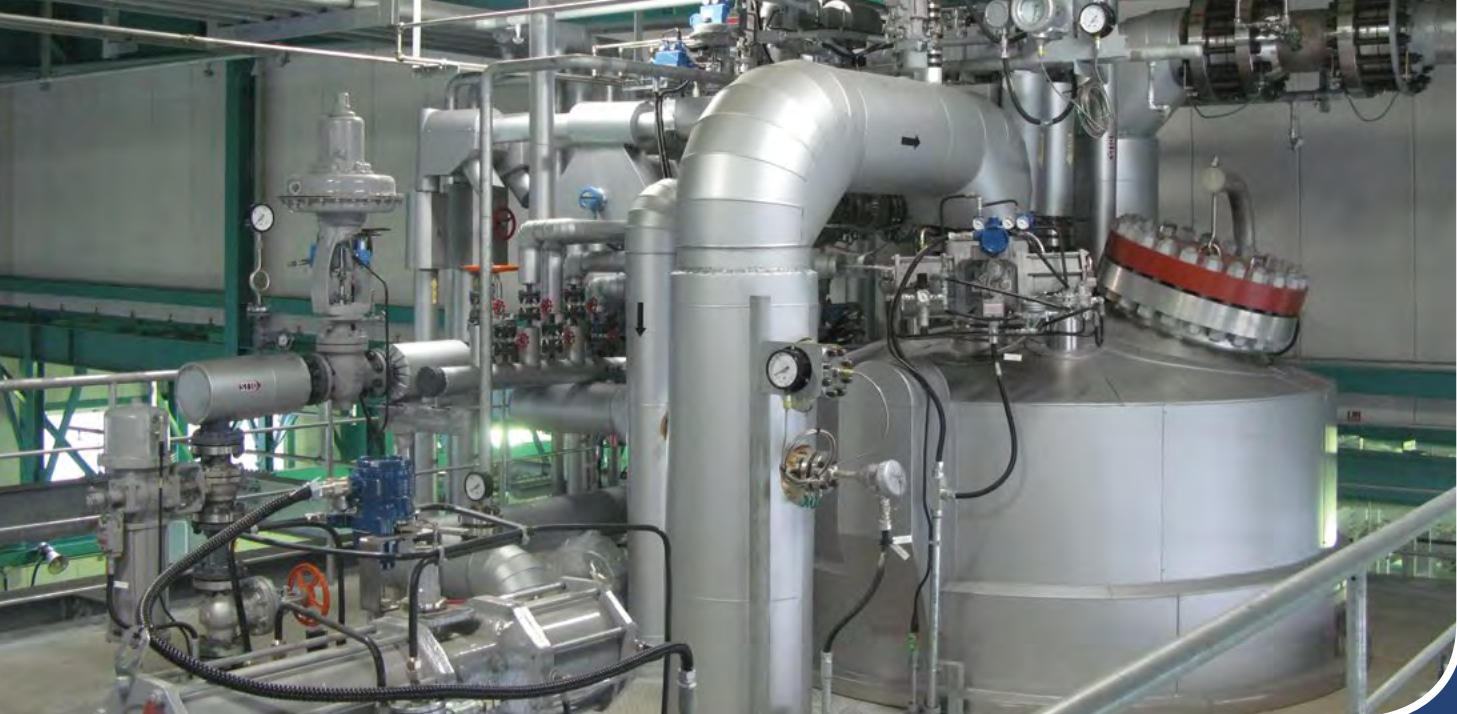
Enhanced Loop Reactor for Ethoxylation
