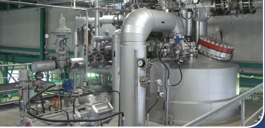
Enhanced Loop Reactor for Ethoxylation
