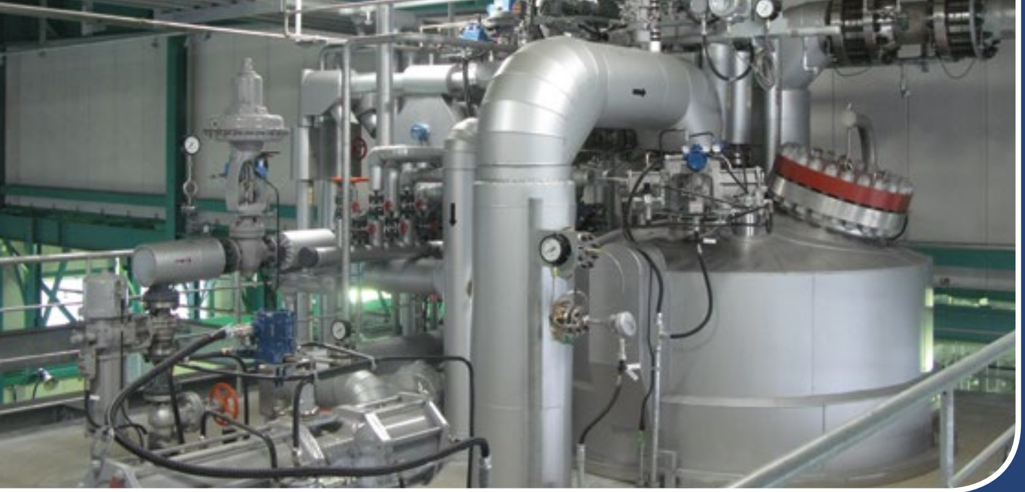
Enhanced Loop Reactor for Ethoxylation
